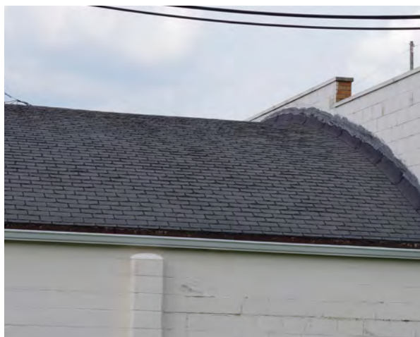
Right: The shingles on the roof of the Moose Lodge are deteriorated. (614 IAA Drive)
