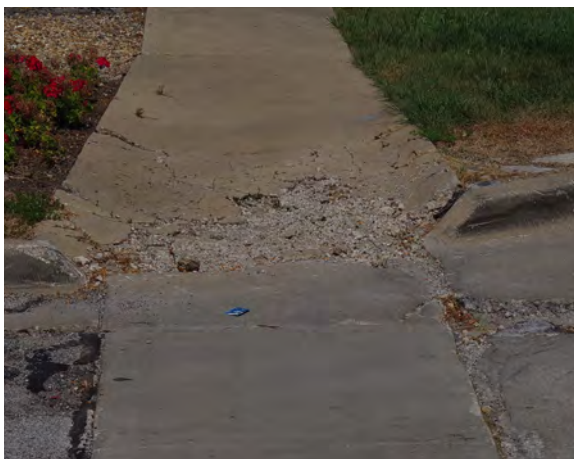
Left: A deteriorated sidewalk along IAA Drive.
