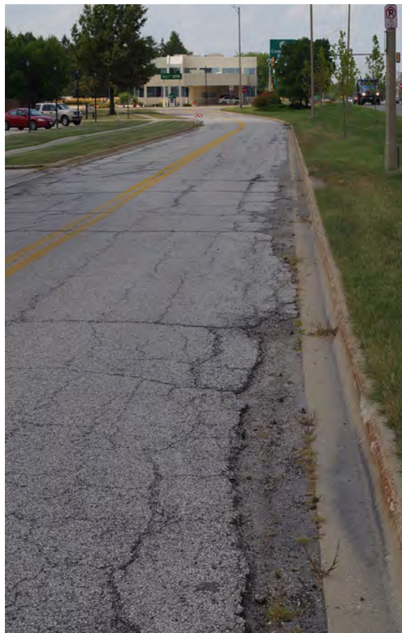
Right: The pavement along Empire Frontage Road South is deteriorated.
