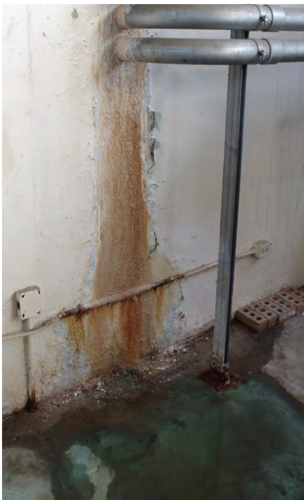
Left: Water seeping through the foundation wall of the boiler room at Bloomington High School. (1200 East Locust Street)
