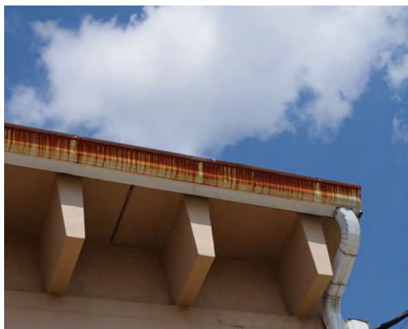
Right: Rust from the roof of the Community Players Theatre is staining the gutters. (201 Robinhood Lane)
