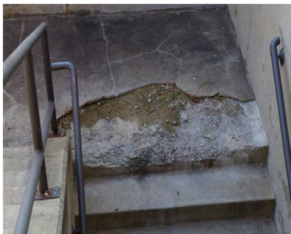
Right: The concrete of this stairwell at Bloomington High School is disintegrating.
