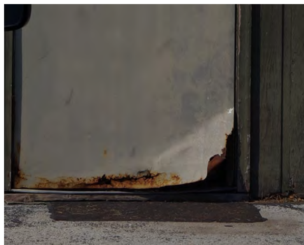
Right: The door on Horine's Piano is deteriorated. (1336 East Empire Street)
