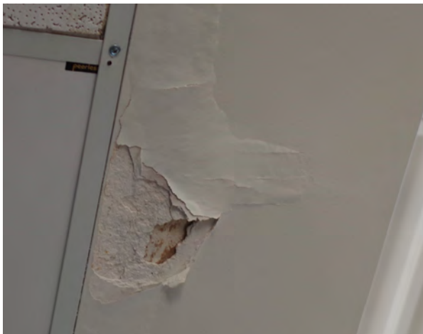
Left: Water damage on the interior of Bloomington High School. (1200 East Locust Street)
