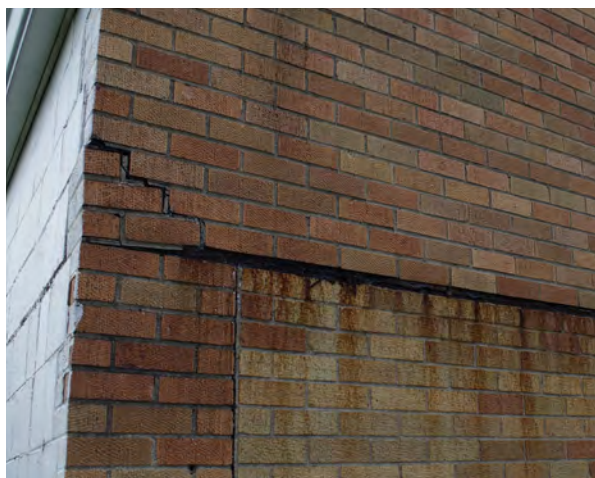
Right: Cracking in the exterior brick wall of the Moose Lodge. (614 IAA Drive)
