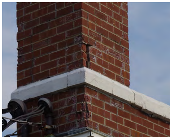
Right: Cracking in the brick chimney of GCE Solutions. (1408 East Empire Street)
