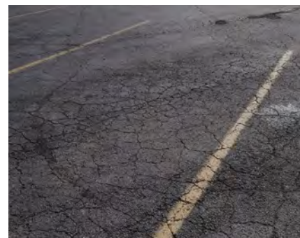
Below: The Arby's parking lot is deteriorated. (1240 East Empire Street)
