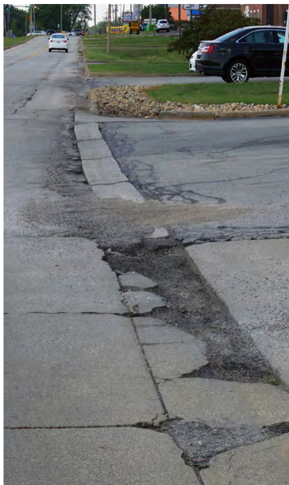
Left: The edge of pavement and the apron entering Colonial Plaza from the south are deteriorated.
