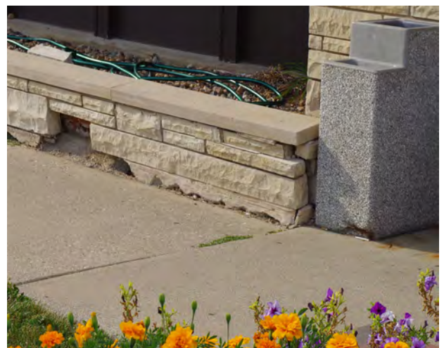
Right: This landscape retaining wall is leaning and deteriorated. (1412 East Empire Street)
