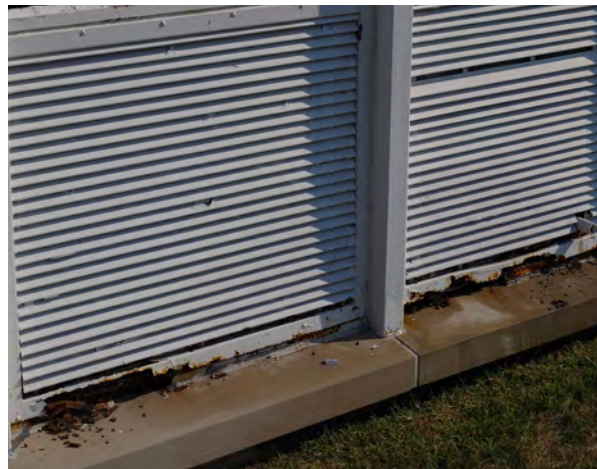
Right: The windows sills at Bloomington High School are rusted and deteriorated. (1200 East Locust Street)
