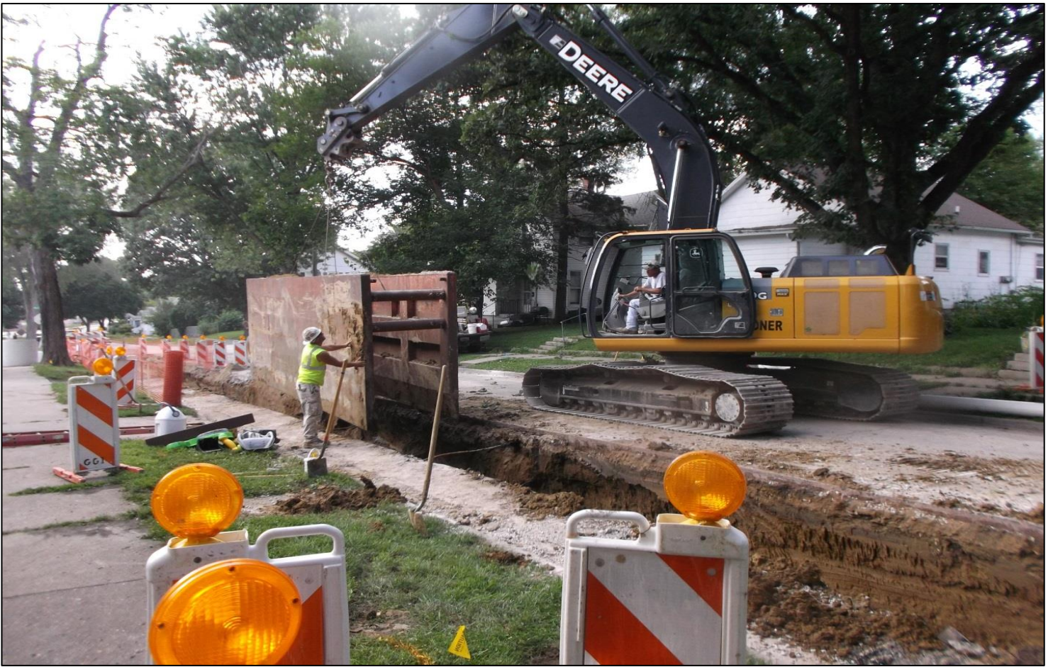
Pictured: Workers from George Gildner Inc. positioned a sewer trench box before laying additional sanitary sewer main in the 500 block of East Jackson Street on July 23.
