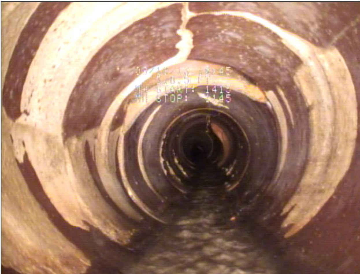
Clayton Street Sewer: Hinge cracking in clay sewer
