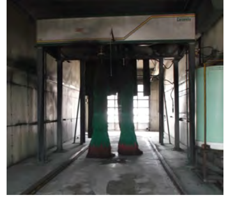
Bus wash (inoperable).
