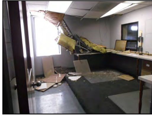
Offices currently unusable.
