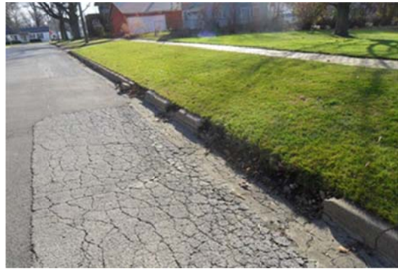
Badly damaged or missing curb pieces must be replaced; adjacent curb remains serviceable.
