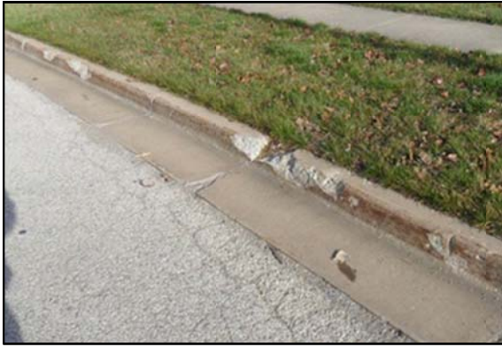
Chipped or spalling curb which remains serviceable usually is left in place.
