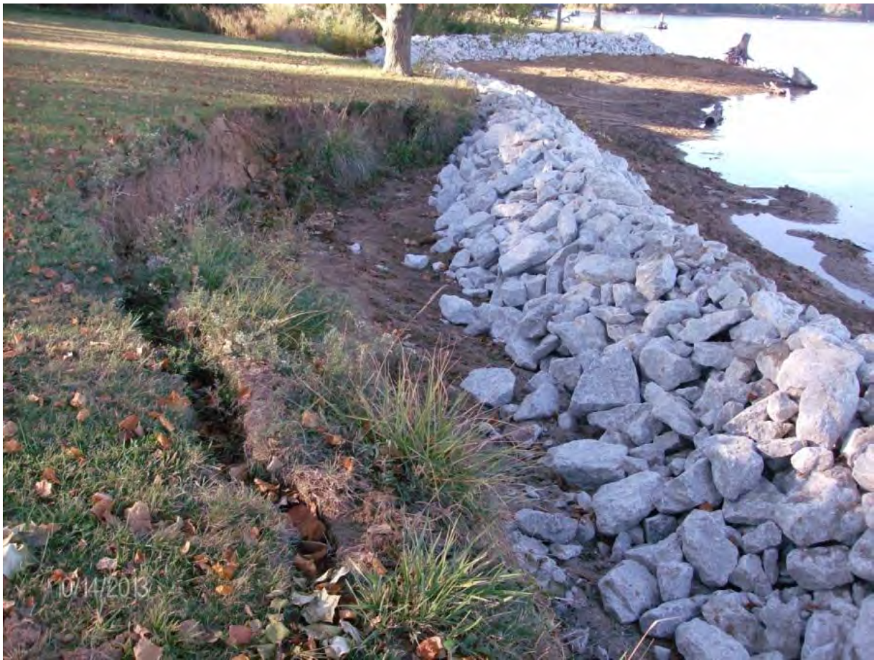
Shoreline protection near the White Oak Boat Ramp (Note pronounced erosion and sloughing of area behind the rip rap)
