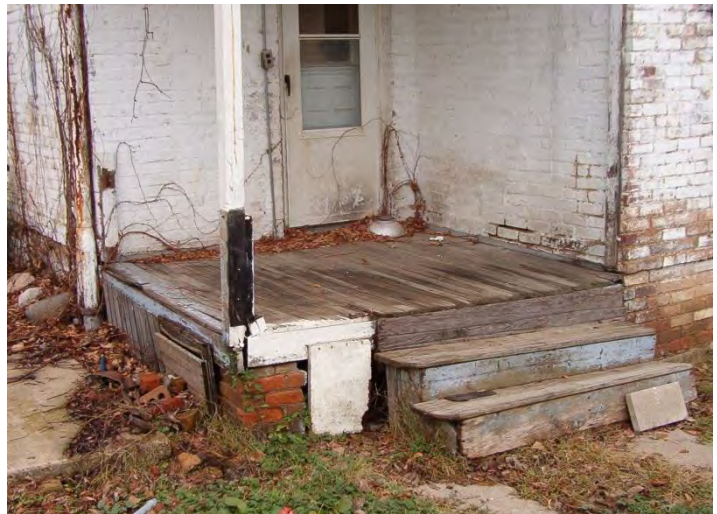
Deteriorated and Unsafe Porch
