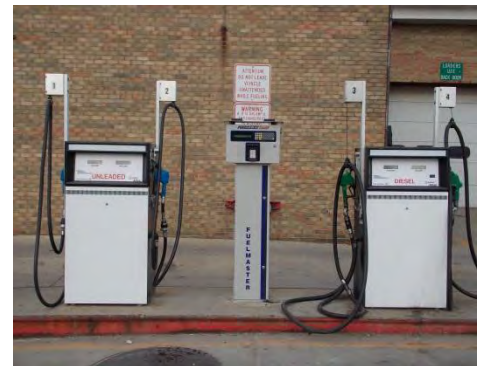
New Fuel Pumps
