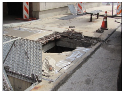
Figure 10: A Collapse Sidewalk Above a Vault
