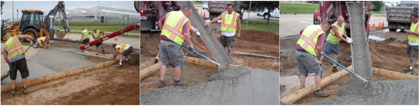
Public Works, Streets Division pours concrete at Fire Station #2 on Hamilton Road
