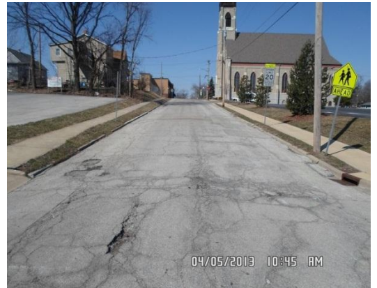
Jackson Street Prior to CRF Treatment
