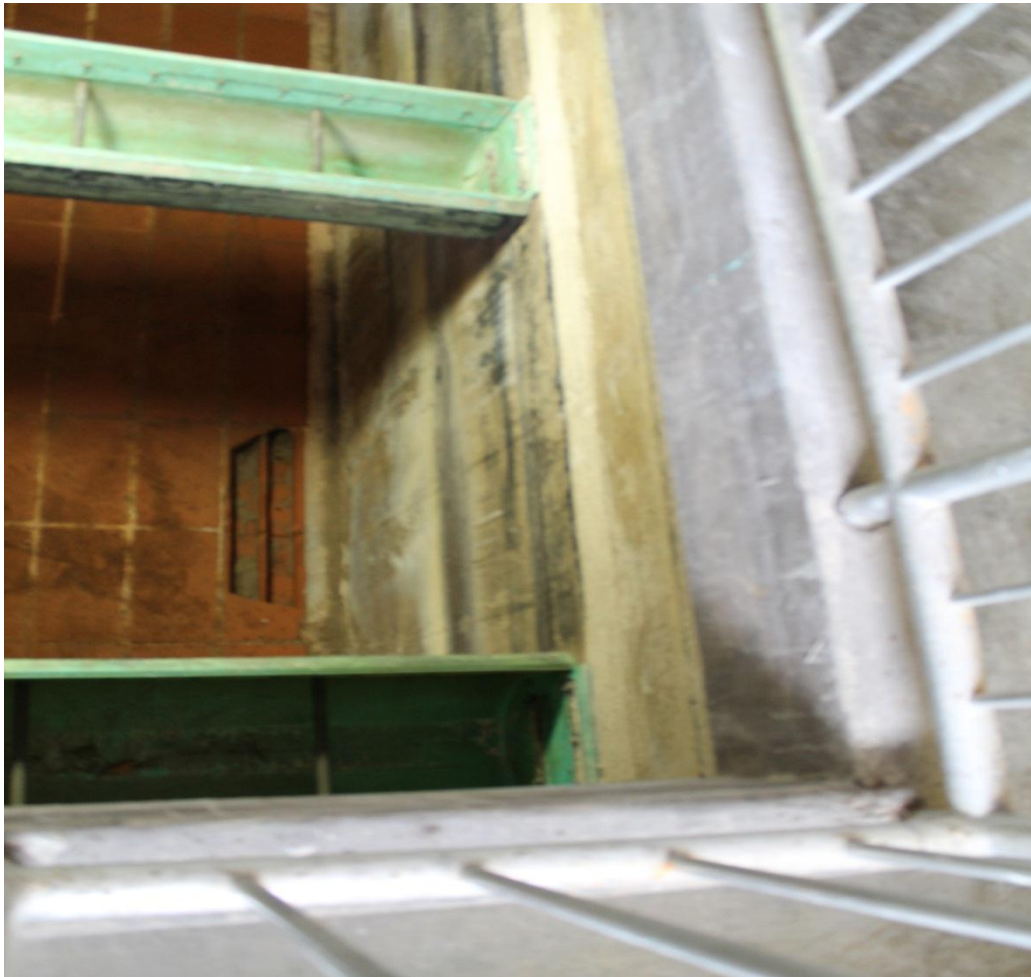
Looking down into empty (filter sand and gravel removed) filter cell the underdrain failure between the two greenish troughs.
