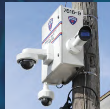
Expanded Public Safety Cameras on intersections using fiber optics
