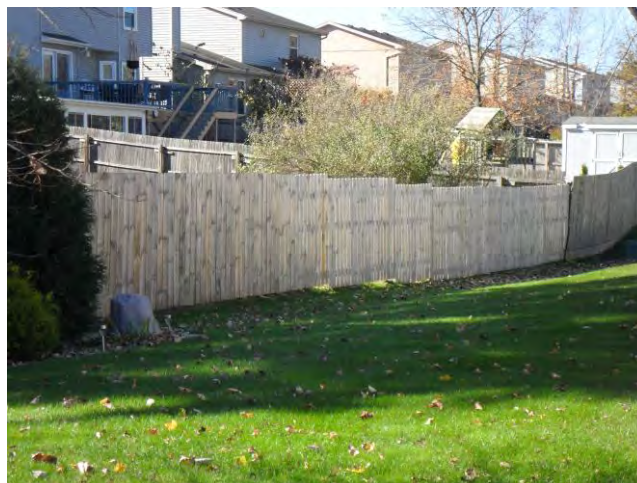
Figure 3: A segment of the perimeter fence adjoining rear and side yard fences to the south.
