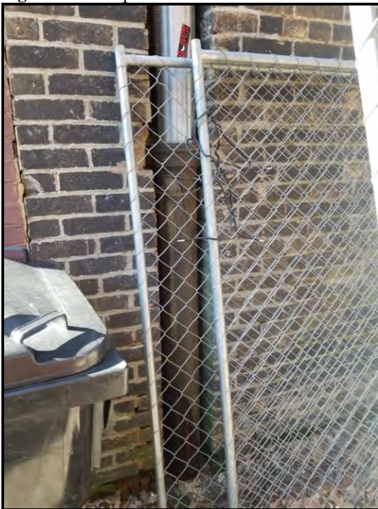
Figure 5 Lower portion of downspout made of cast iron to be replaced.
