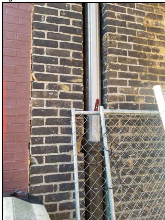
Figure 3 Downspout on the rear elevation located in the alley showing the transition from steel to the cast iron portion to be replaced.
