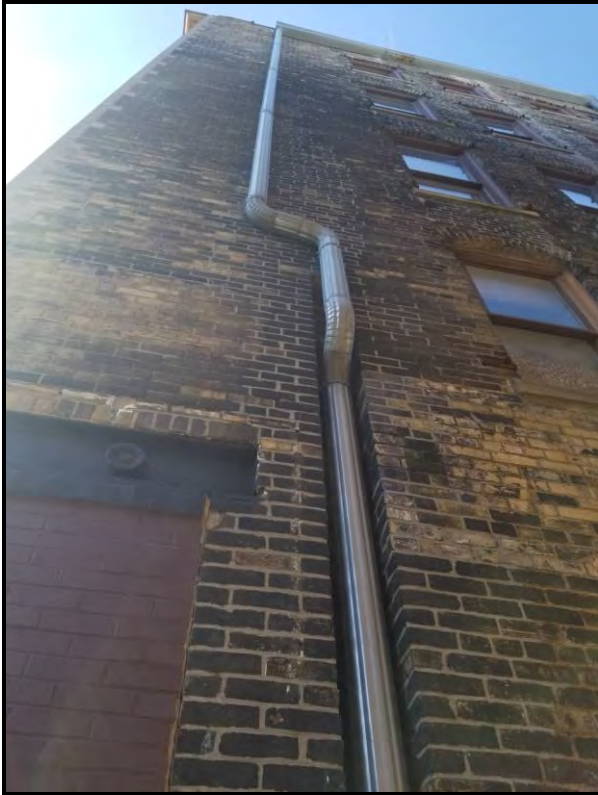
Figure 4 Downspout located on the rear elevation in the alley leading to the cast iron downspout to be replaced.
