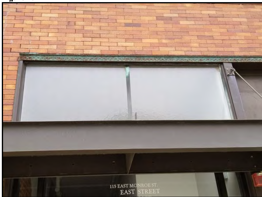
Figure 11 Photo showing detail at the top of the transom window above the east entrance pictured in Figure 10
