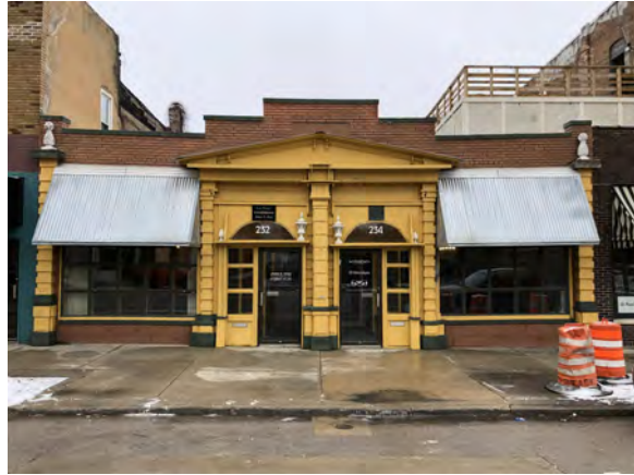
OVERALL VIEW OF EXISTING WOOD CLADDING FACADE WITH ORIGINAL FACE BRICK BEYOND.
