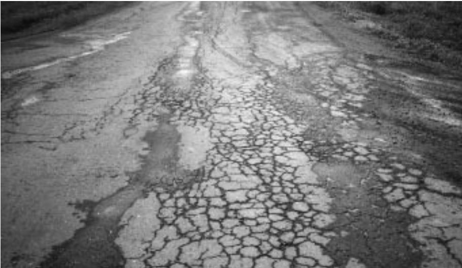
◀ Characteristic "chicken wire" crack pattern shows smaller pavement pieces and patching.
