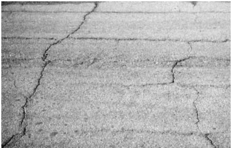
▶ Intermediate-size block cracking, 1'-5' across with open cracks.
