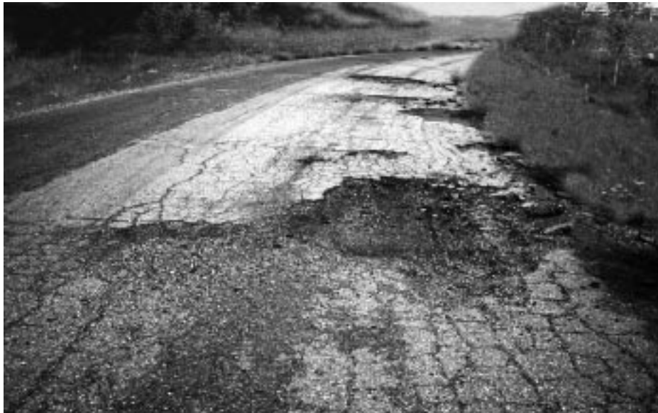
◀ Large, isolated pothole, extends through base. Note adjacent alligator cracks which commonly deteriorate into potholes.
