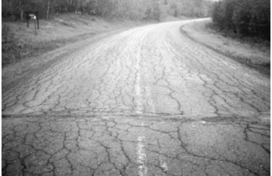
► Extensive alligator cracking. Pulverize and rebuild.
