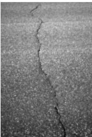
▲ Tight cracks less than 1/4" in width.
