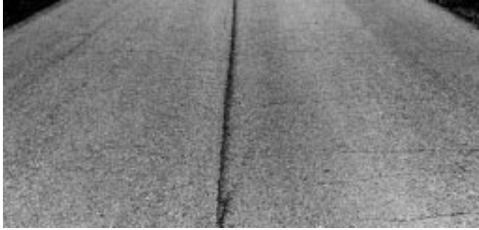
Centerline crack (still tight). ▶
