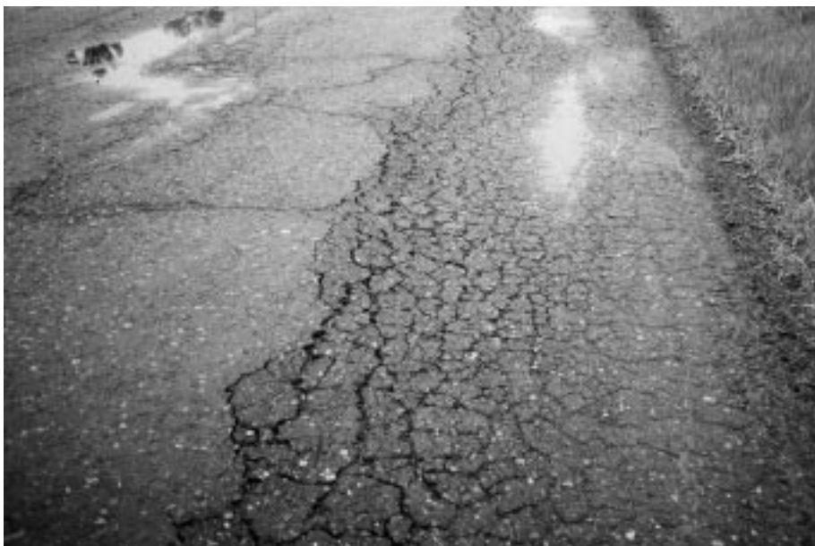
◀ Open raveled alligator cracking with settlement along lane edge most likely due to very soft subgrade.
