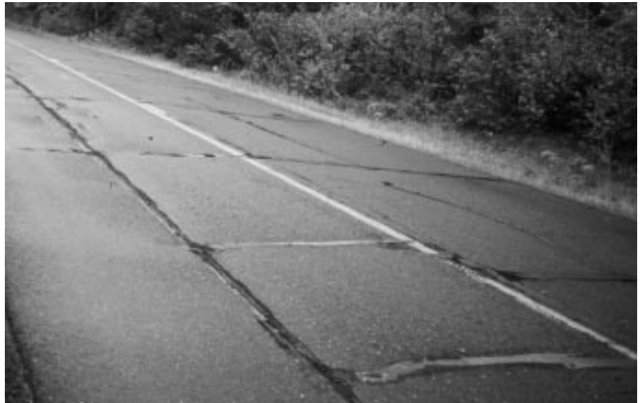
► Concrete joints reflected through bituminous overlay.
