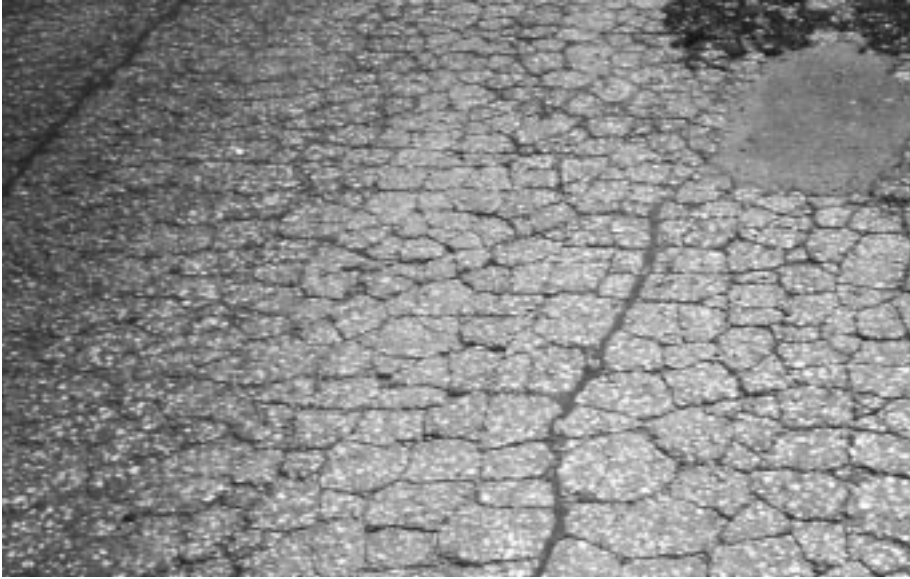
◀ Alligator crack pattern. Tight cracks and one patch.
