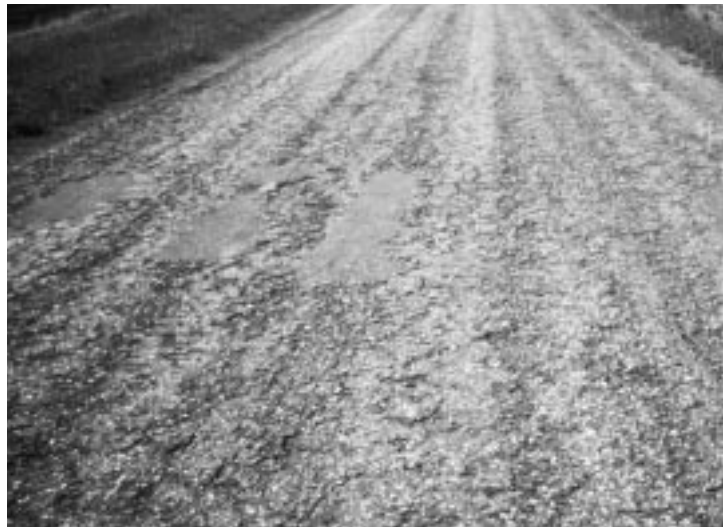
◀ Severe raveling and loss of surface material.
