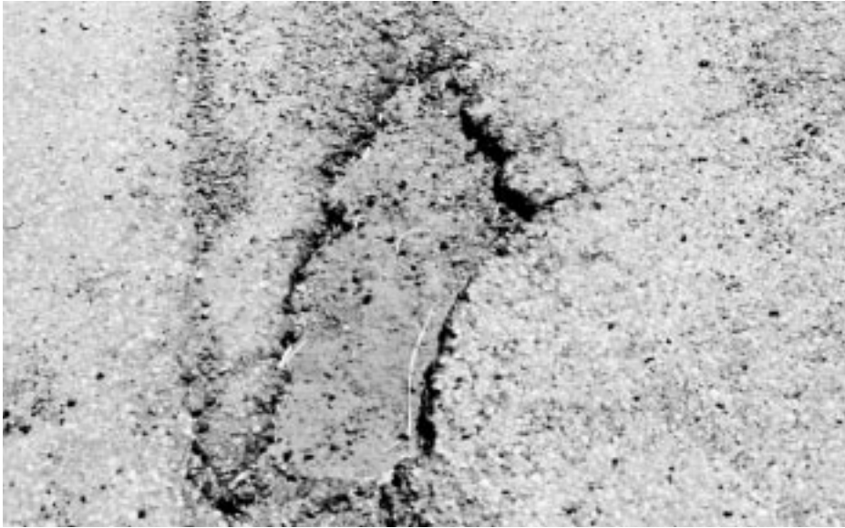
◀ Small pothole where top course has broken away.
