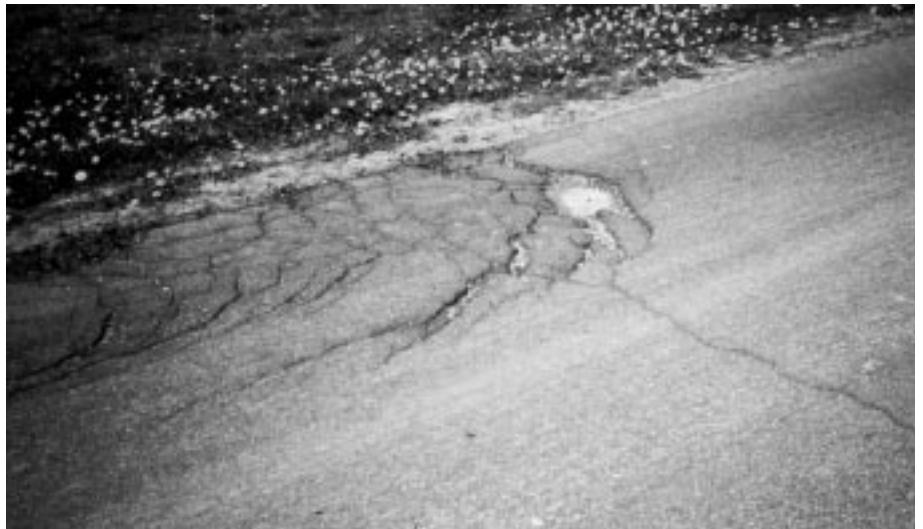
► Crescent-shaped cracks characteristic of slippage.
