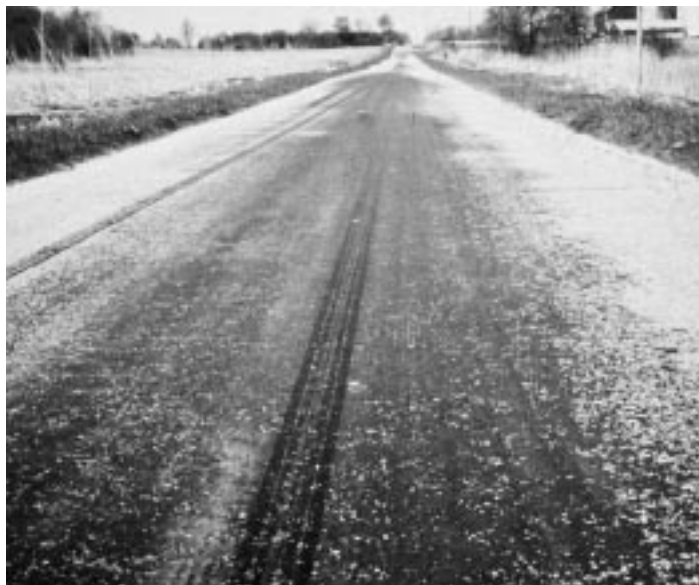
▶ Flushing. Dark patches show where asphalt has worked to surface.
