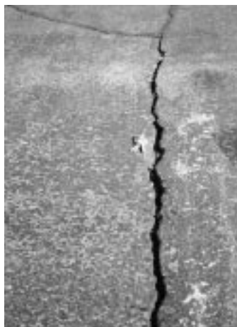
▲ Open crack – 1/2" or more in width.
