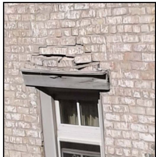
Window needing repair at 411 N Center
