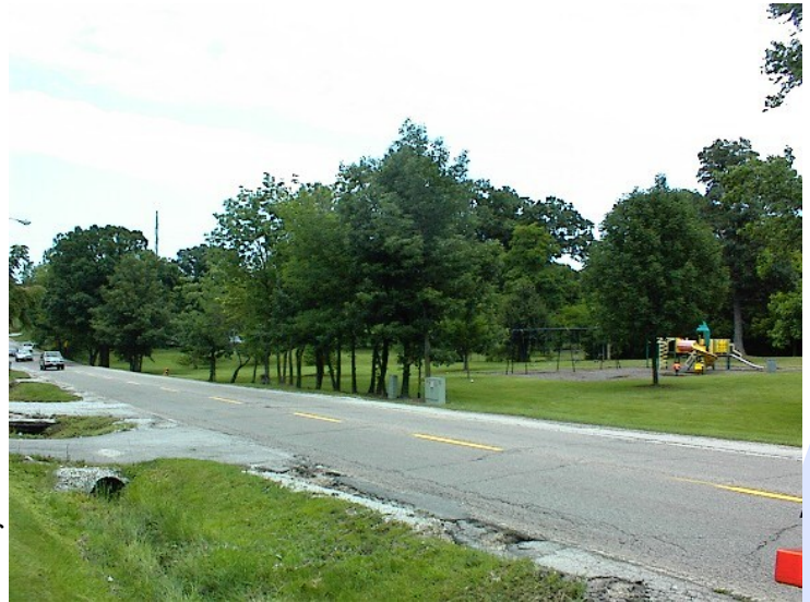
Existing 2 lane section of Morris Avenue near Miller Park Zoo with cracking asphalt and open storm water ditches
