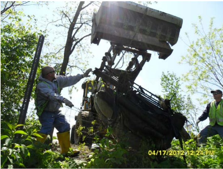
City of Bloomington Local 699 Employees, Aaron Barlow and Joe DeGraeve work with an End Loader to pull furniture from the lake.
