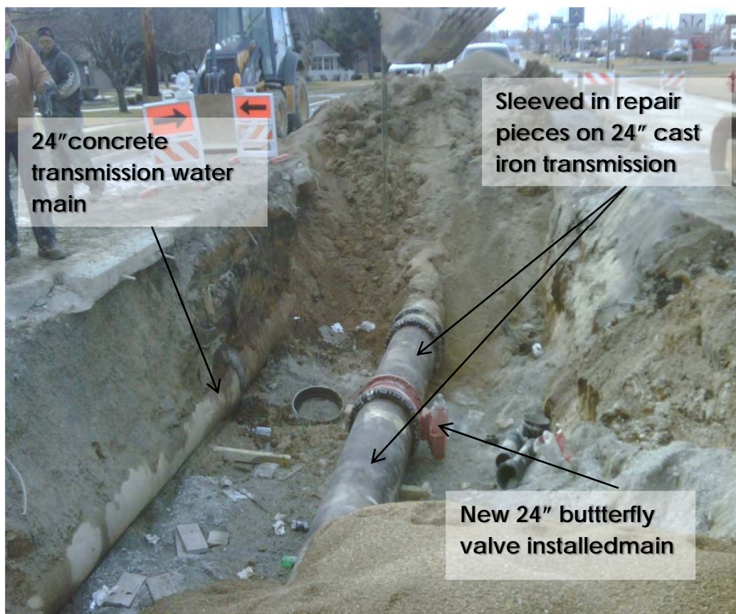
24" cast iron water main repair on Fort Jesse Road – looking west towards Towanda Avenue
