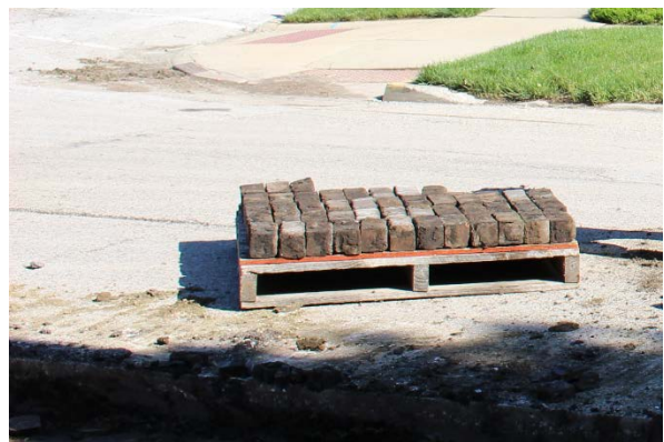
6. Carefully stack undamaged bricks on a pallet on location or at another location, depending on the method used. Count on having to discard 30 percent of the bricks because of various types of damage.
