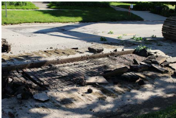
3. Clean residual asphalt from the bricks. Power washing is a common method.
