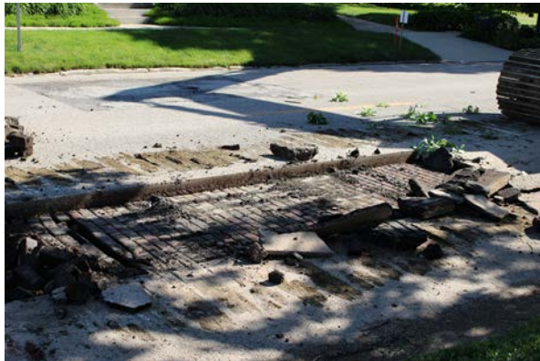
3. Clean residual asphalt from the bricks. Power washing is a common method.
