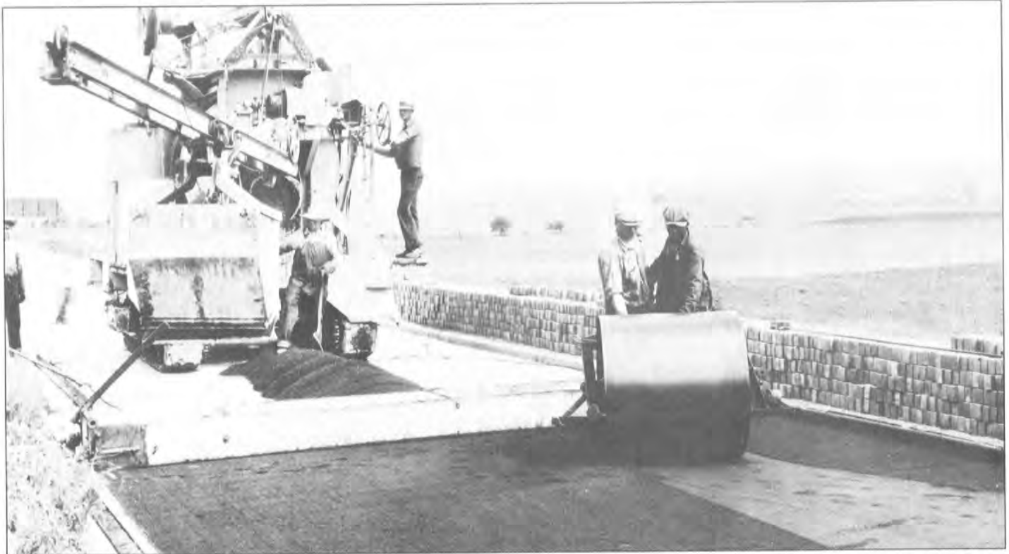
Above: Workers prepare the foundation for a brick pavement in rural McLean County about 1925. Photo: McLean County Historical Society. Below: The November 1916 Issue of Dependable Highways featured a crew setting bricks on a prepared foundation.
