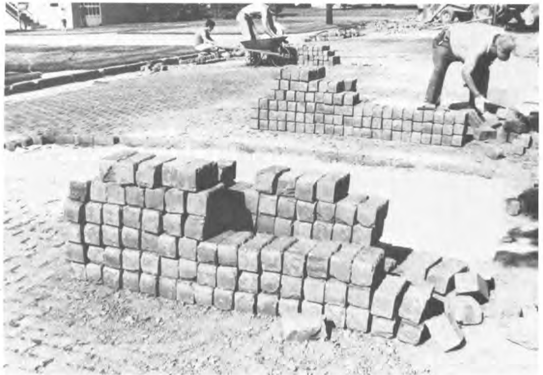
Author Royce Baier (center) in 1990 leads a work crew on the restoration of East State Street in Paxton. Photo by Ralph Schmanski
