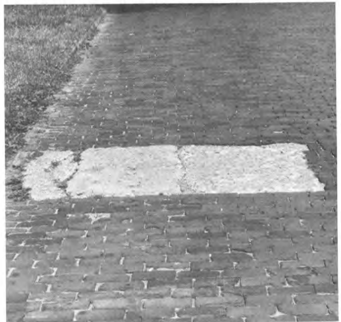
A typical concrete-patched utility cut. Photo by Chris Harbison
