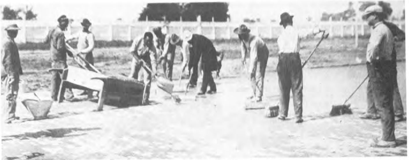
Installation of a wet cement-sand filler. Brooms and squeegees are used to fill the joints and clean the surface of the brick. This photograph appeared in Dependable Highways.
