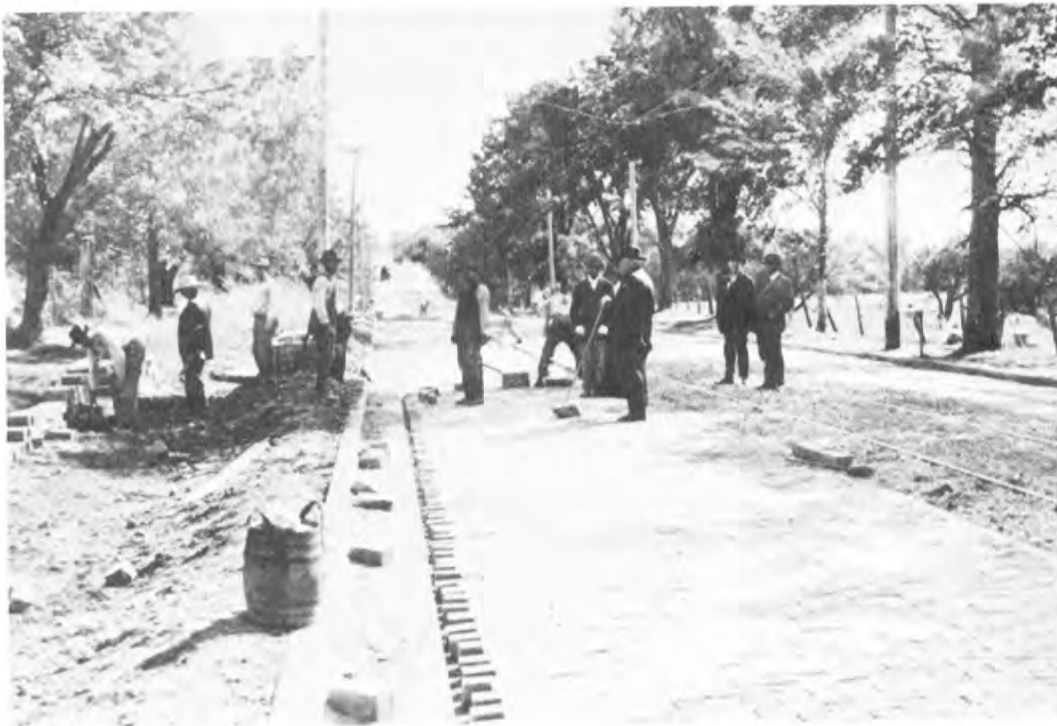
The last step in laying a brick pavement, shown in Dependable Highways, is setting the cut bricks at the curb. There, bricks are custom-cut to fit the gap. These workers are constructing the Lincoln Highway in Dixon.
