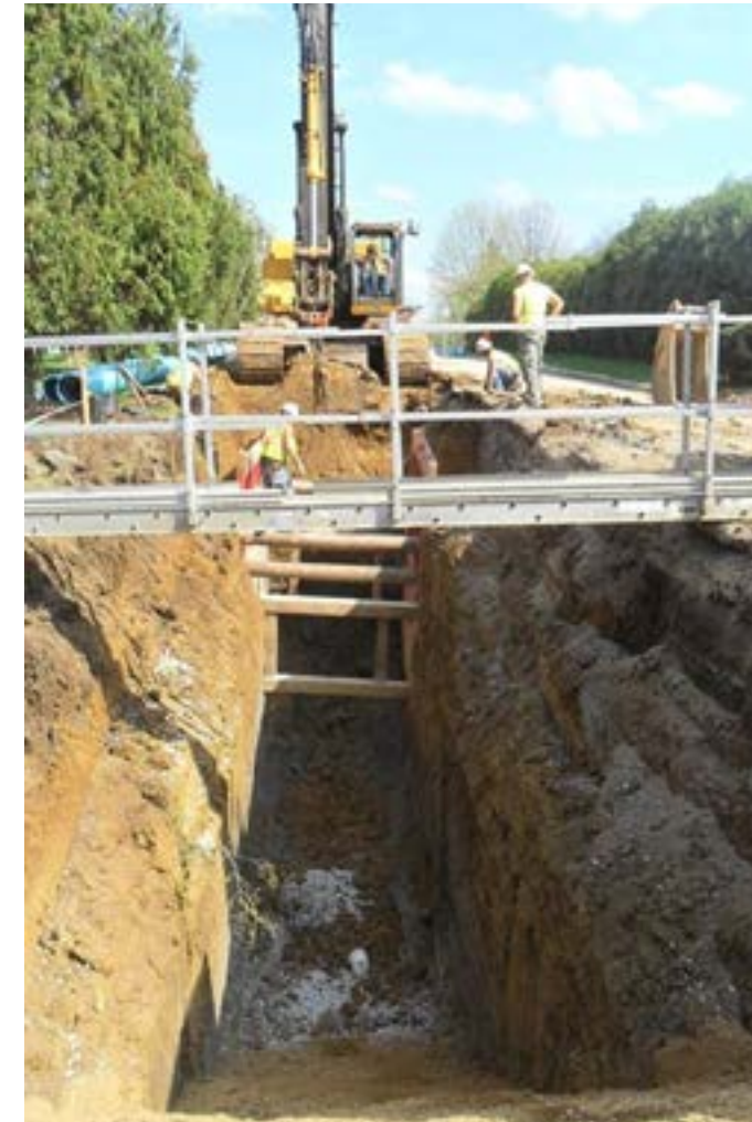
Figure 10-1. Department of Public Works project at a combined sewer overflow location Source: City of Bloomington Department of Public Works
