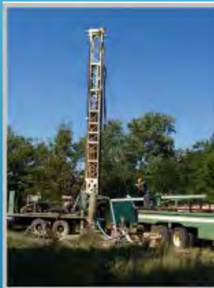
Southwest Well Field
